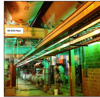
NitRAS underground pipe gallery conditions at Blue Plains AWTP. Photo courtesy of DC Water.
